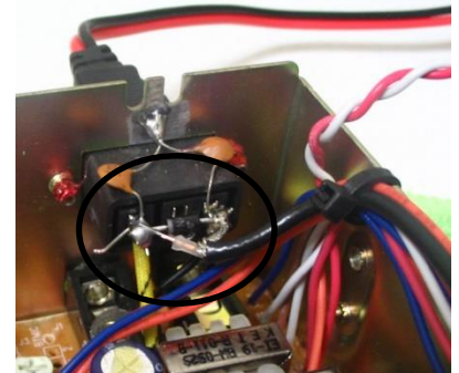
Typical power cable connection.
